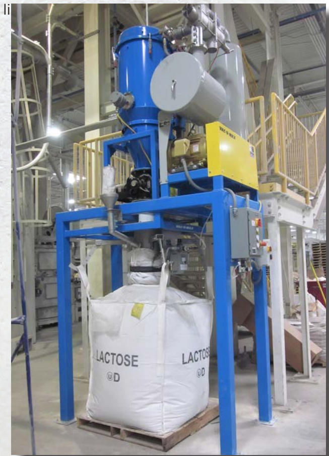
Central vacuum cleaning system with source capture and reclaim into bulk bag for potential reuse, recycle, or disposal.
